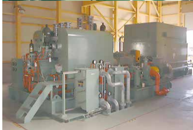
17,800kW Extraction (controlled) back pressure Turbine for Co-generation Power Plant, Oita Factory of Oji Craft Paper Corporation
