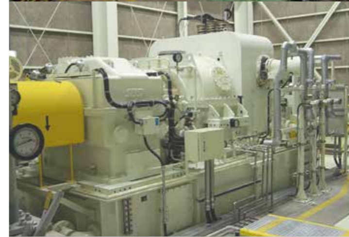
4,200kW Extraction (bleeding) Condensing Turbine for Gas Turbine Combined Cycle Power Plant, Miyoshi Factory of Toyota Motor Corporation
