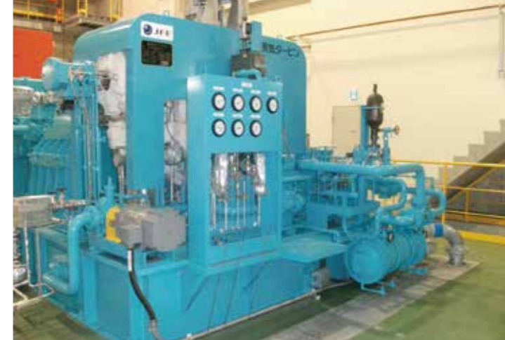
9,700kW Extraction (bleeding) Condensing Turbine for Clean Plaza Fujimi (municipality), Tokyo
