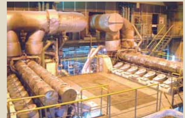
Electric power plant (14PC2-6V)
