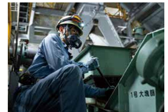
Mechanical Equipment Inspection and Maintenance
